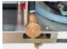
UNI 45 water hydrant connection
